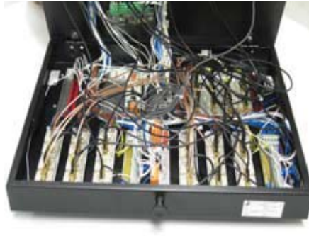
Fixtures enclosure with a lot of free space to include special custom test assemblies
