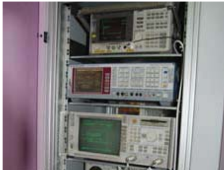
High rack space for test instruments and ease cables layout.
